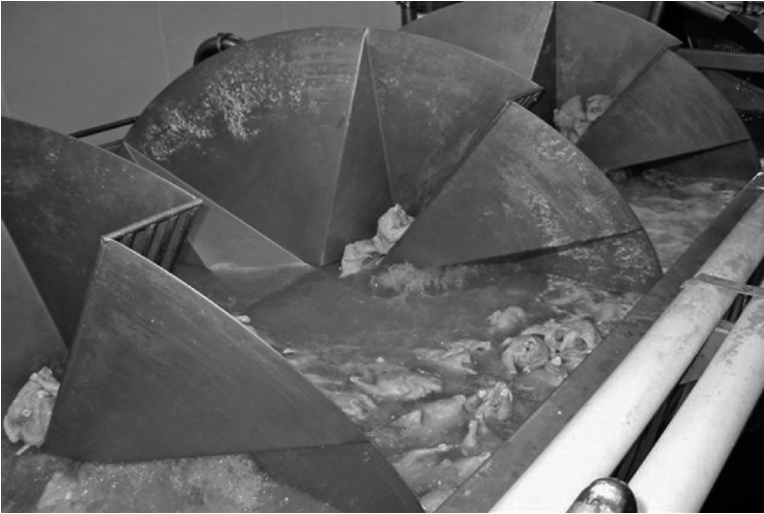
Figure 21.6 This is a chiller in El Salvador that is operating properly with extremely clean water containing very low organic loading.
