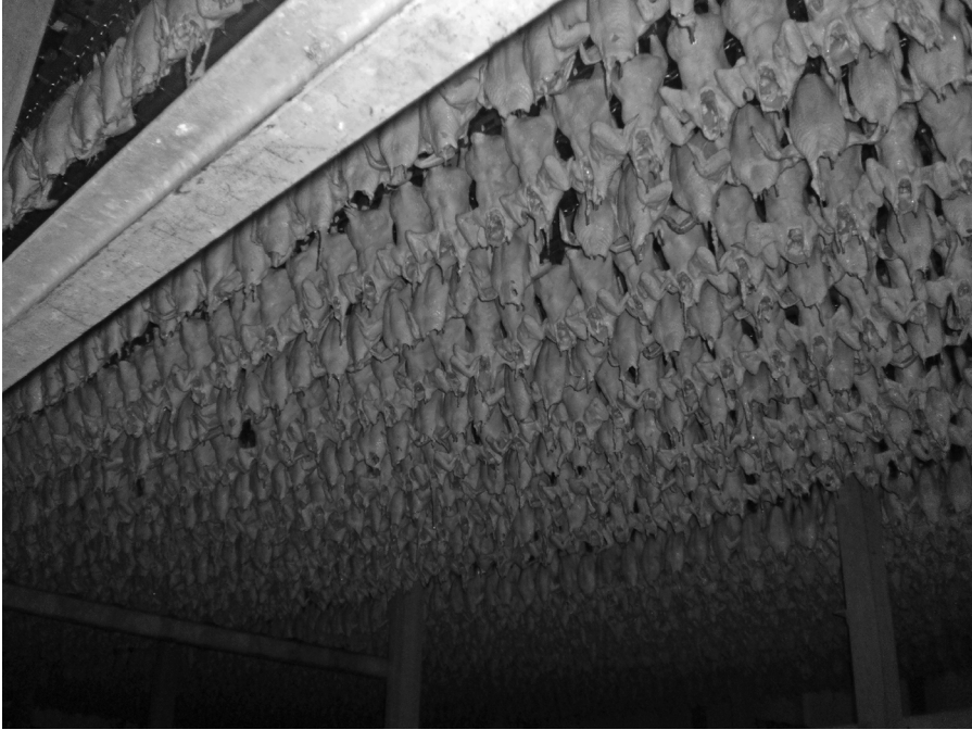
Figure 28.3 Typical air chiller used in the European Union.
