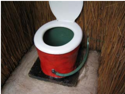
Figure 6-31: Urine-diverting pedestal installed
