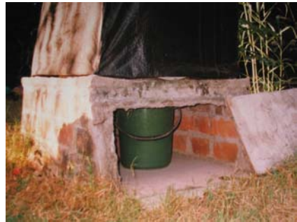
Figure 6-40: Internal view of vault with plastic bucket placed for collection of faeces
