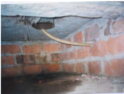
Figure 6-37: Plastic pipe carries urine from the urine-diverting pedestal
