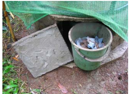
Figure 7-6: Concrete vault access door
