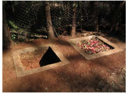
Figure 6-50: Twin pits ready for use with right-side pit filled with leaves
