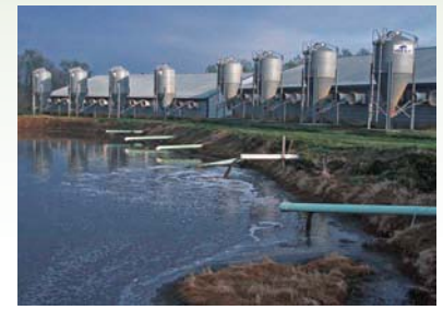
Figure 4-7 A state of the art lagoon waste management system. This facility is highly automated and is temperature controlled. Courtesy of USDA Natural Resources Conservation Service. Photo by Jeff Vanuga.
