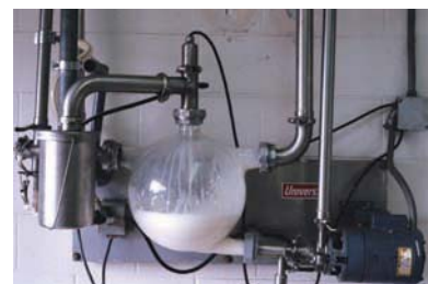
Figure 43-3 Milk flows down the pipeline into a holding tank, then into a bulk tank for cooling and storage. Courtesy of Getty Images.
