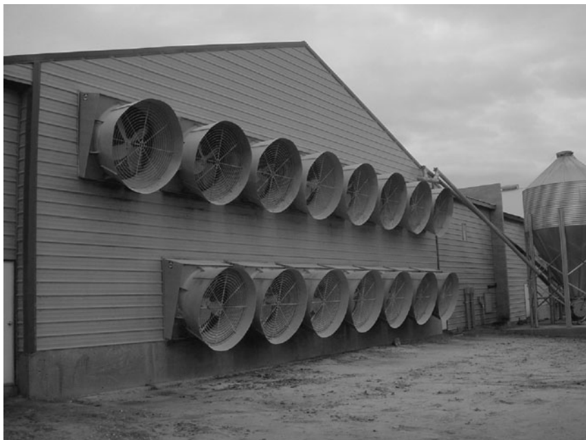
Bi-directional tunnel-ventilated house with fans.
