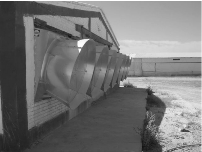
Fig. 5.31. Discharge cone fans.
