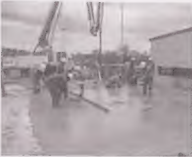
FIG. 3—Construction of the base for a heat-treating facility in Houston, TX. Cycling of temperatures caused severe breakdown of conventional concrete [18].
