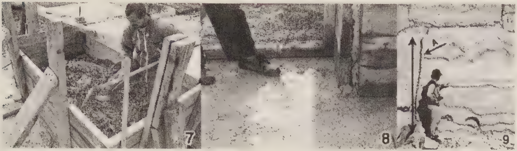
Figure 10.9: Failure. 7. The mixture containing too much water becomes muddy and a man sinks down. 8. The pressure on the liquid paste is transmitted to the mould whose sides pull apart at the ends. Excess water drips out. 9. This produces curved edges identical to those found on the large blocks of the pyramid of Chephren. The Egyptians had to deal with the same problems as us.
