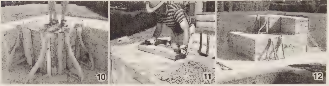
Figure 10.10: From packing to releasing: five blocks totalling 12.2 tonnes of natural limestone. 10. Like adobe, the material is packed with a pestle. 11. The surface is smoothed and levelled with a length of plank. 12. After three weeks, the limestone of the two 4.5-tonne blocks forming the base is strong enough to support the next layer, comprising two blocks of 1.5 tonnes and 1 tonne. The fifth block of 750 kg (in the centre of the second tier) is packed into the mould made from small planks supported by "Egyptian" stays.
